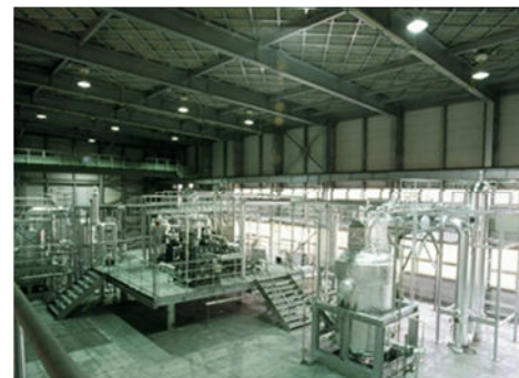
Figure 3: 30 kW OTEC and Desalination Room, Saga-Japan [IOES]
