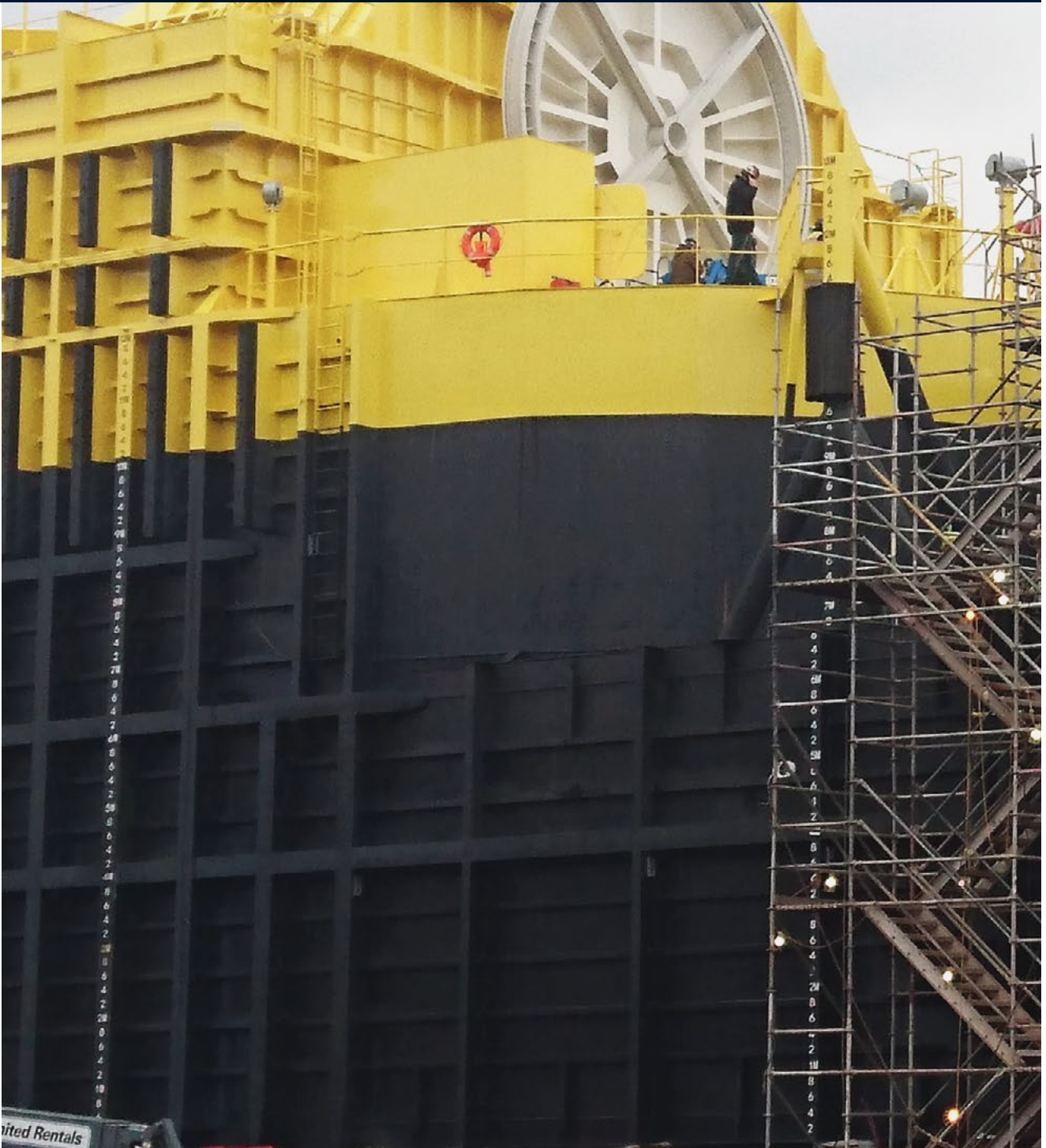
OE35 Buoy under construction at an Oregon shipyard before being towed to the US Navy Wave Energy Test Site, in Hawaii Courtesy: Ocean Energy Ltd
