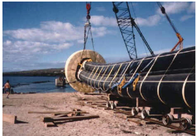
Figure 4.3 Horizontal launch of the OTEC-1 cold water three pipe bundle, Big Island of Hawaii
