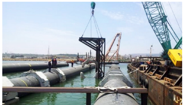
Figure 8.3 Concrete collars on a 2.5m water intake pipeline, Ras Djinet Gas Turbine Power Plant, Algeria
